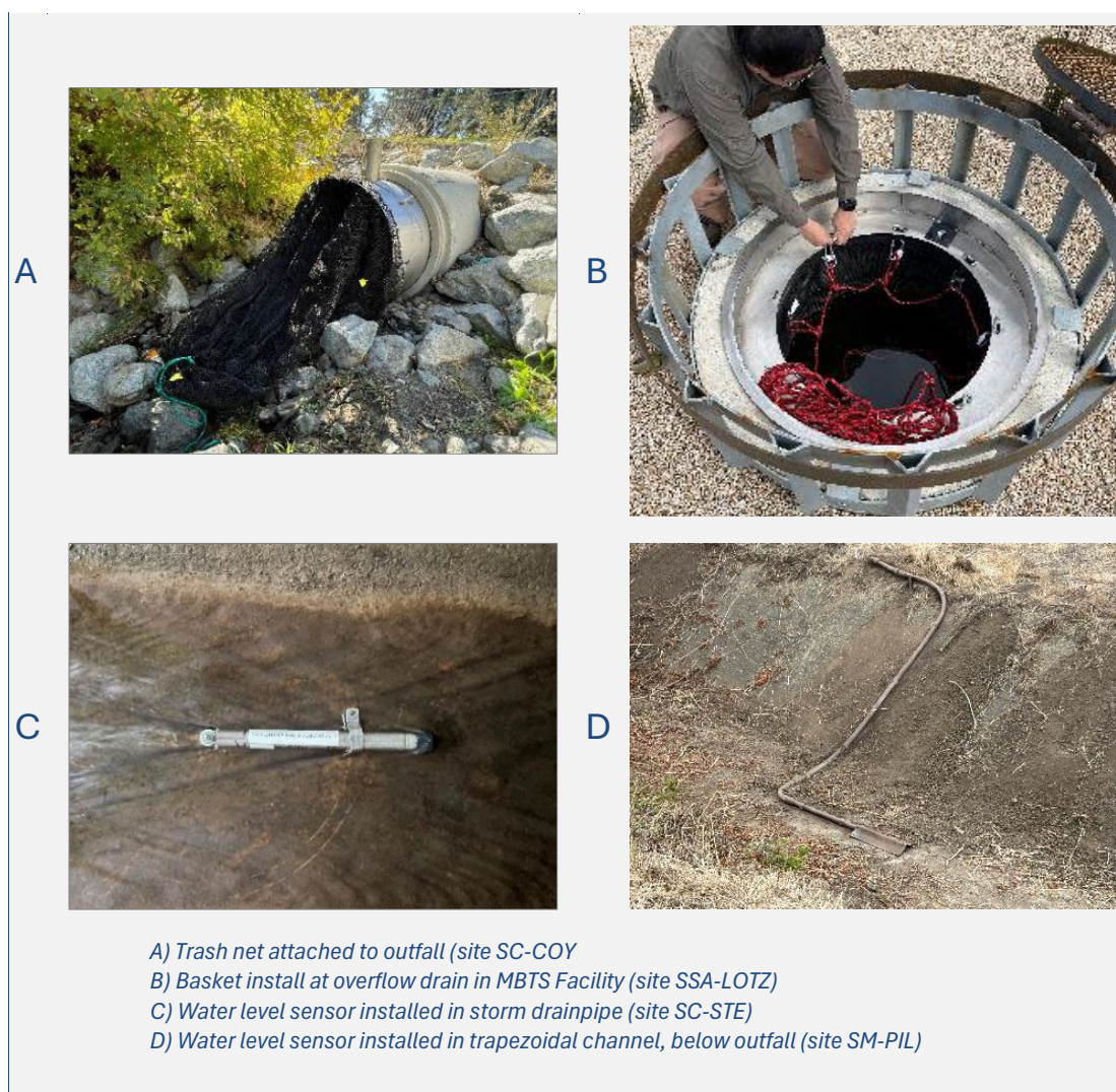
Figure 2. Monitoring equipment is installed at storm drain outfalls.
