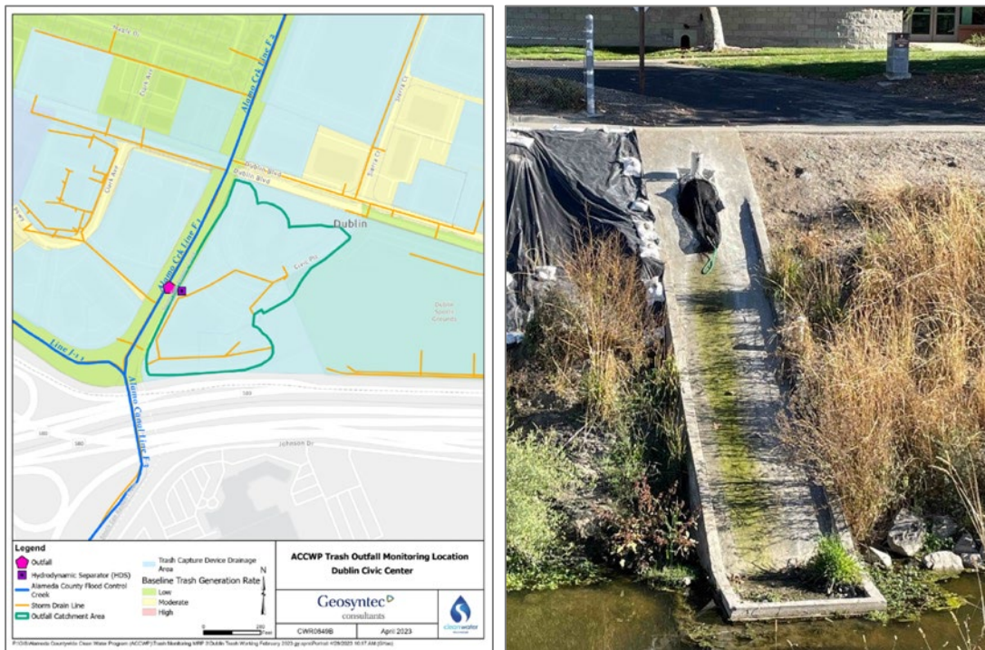
Figure AC-5. AC-CIVIC outfall, with the NetTech™ monitoring device, located on the east bank of Alamo Canal, City of Dublin
