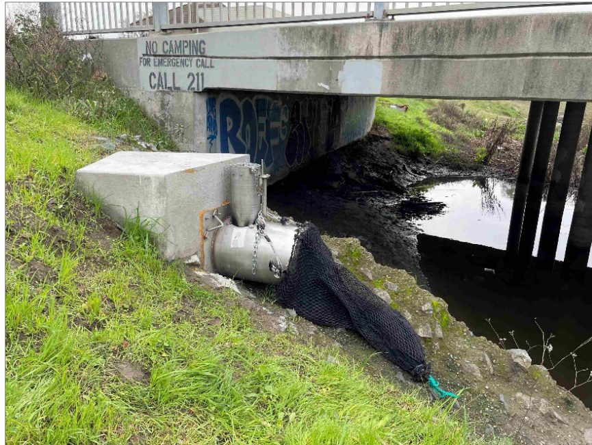
Figure CC-3. Trash monitoring outfall located in census designated place of Pacheco, Contra Costa County
