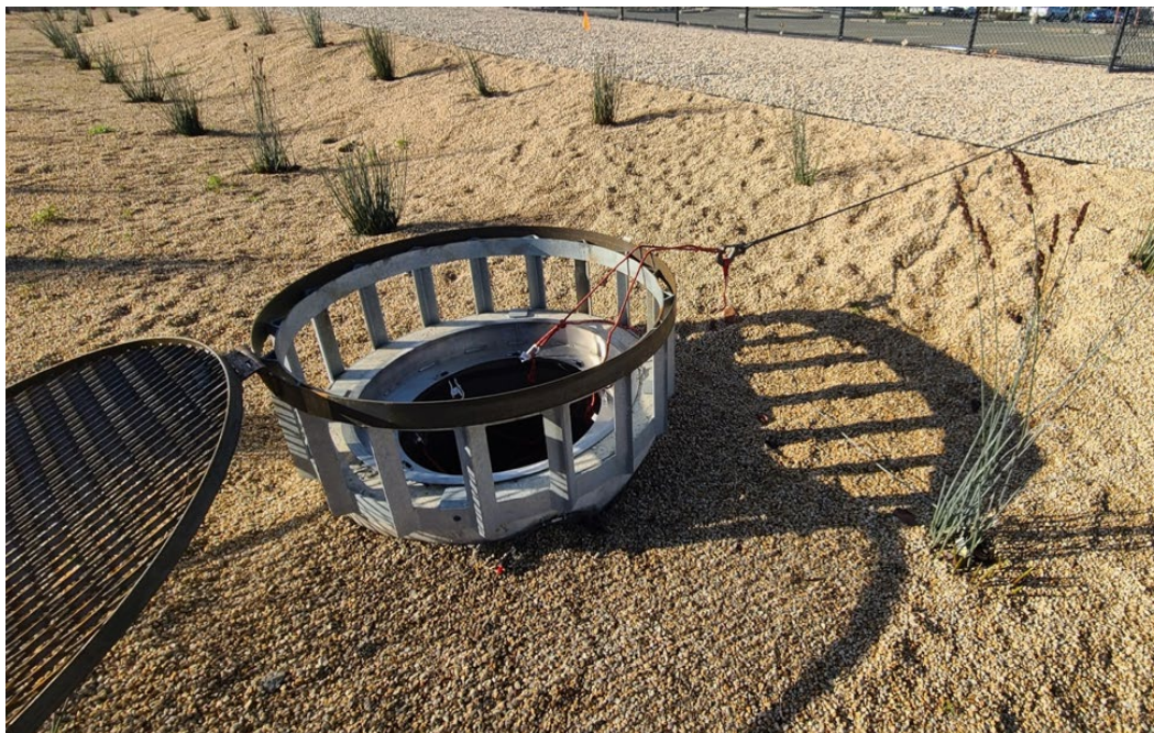
Figure SSA-3. Amtrak Park & Ride MBTS overflow with trash capture net installed
