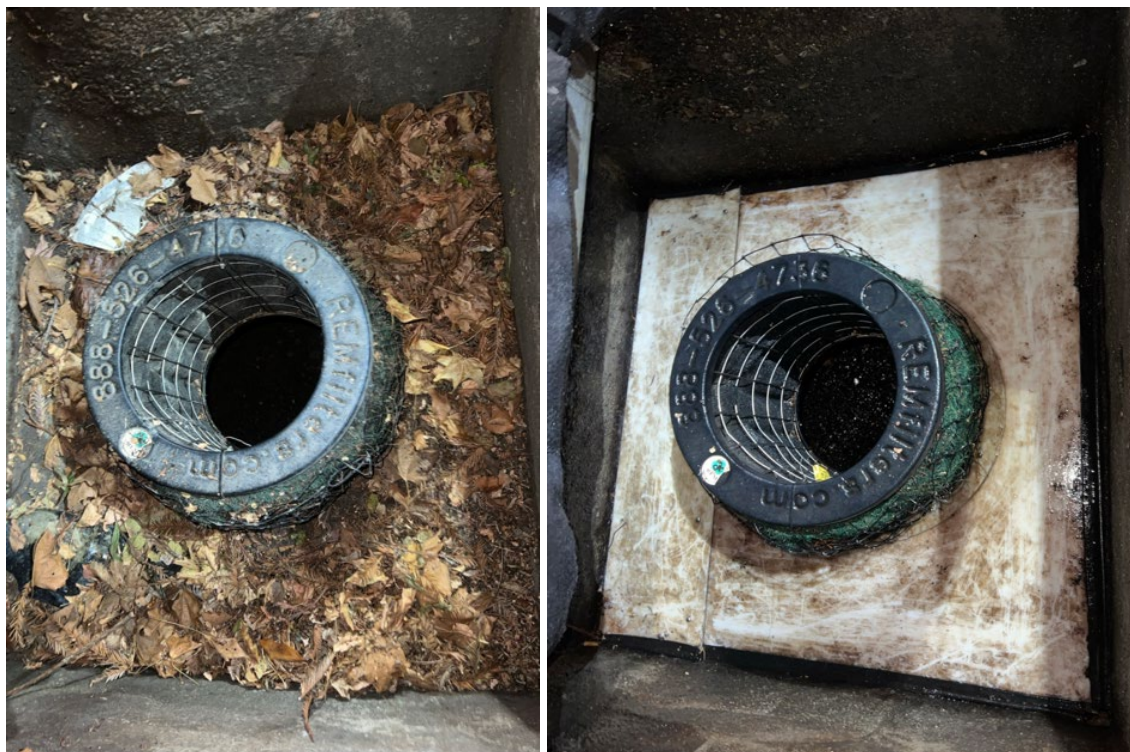
Figure AC-33. Photos of City of Dublin catch basin insert DUB-FCD-059 before (l) and after (r) cleaning event on November 4, 2024
