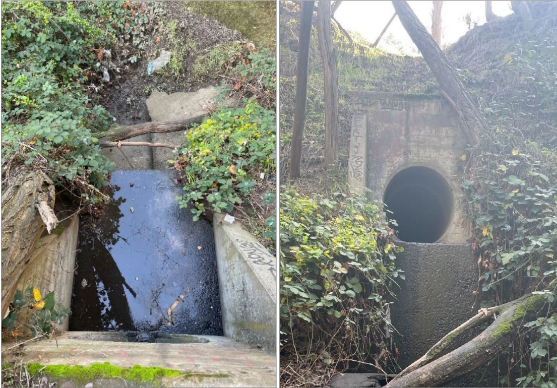
Figure SC-4. Outfall located above San Francisquito Creek, City of Palo Alto
