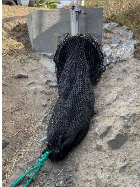
Figure CC-4. Outfall retrofit and netting device install at Grayson Creek outfall site CC-PCH
