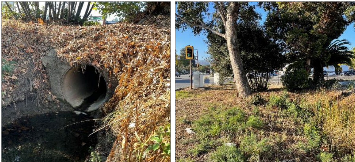
Figure SM-3. Outfall located upstream of drainage ditch to Steinberger Slough, City of San Carlos
