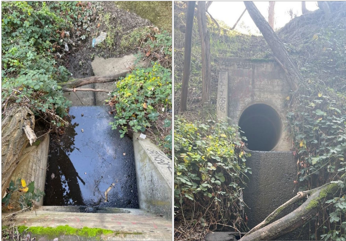
Figure SC-2. Outfall located above San Francisquito Creek, City of Palo Alto
