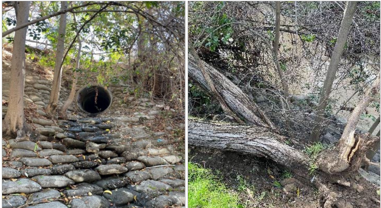
Figure SC-3. Outfall above Stevens Creek, City of Mountain View
