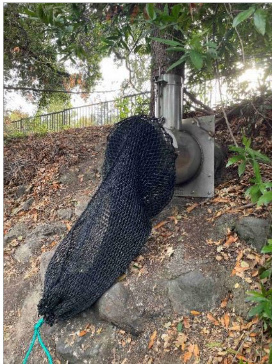
Figure CC-5. Outfall retrofit and netting device install at Walnut Creek outfall at site CC-WC
