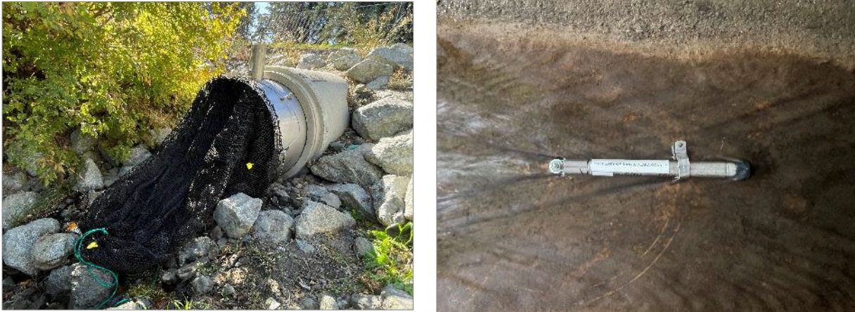
Figure 2. Monitoring equipment installed at each storm drain outfall monitored in WY 2024
