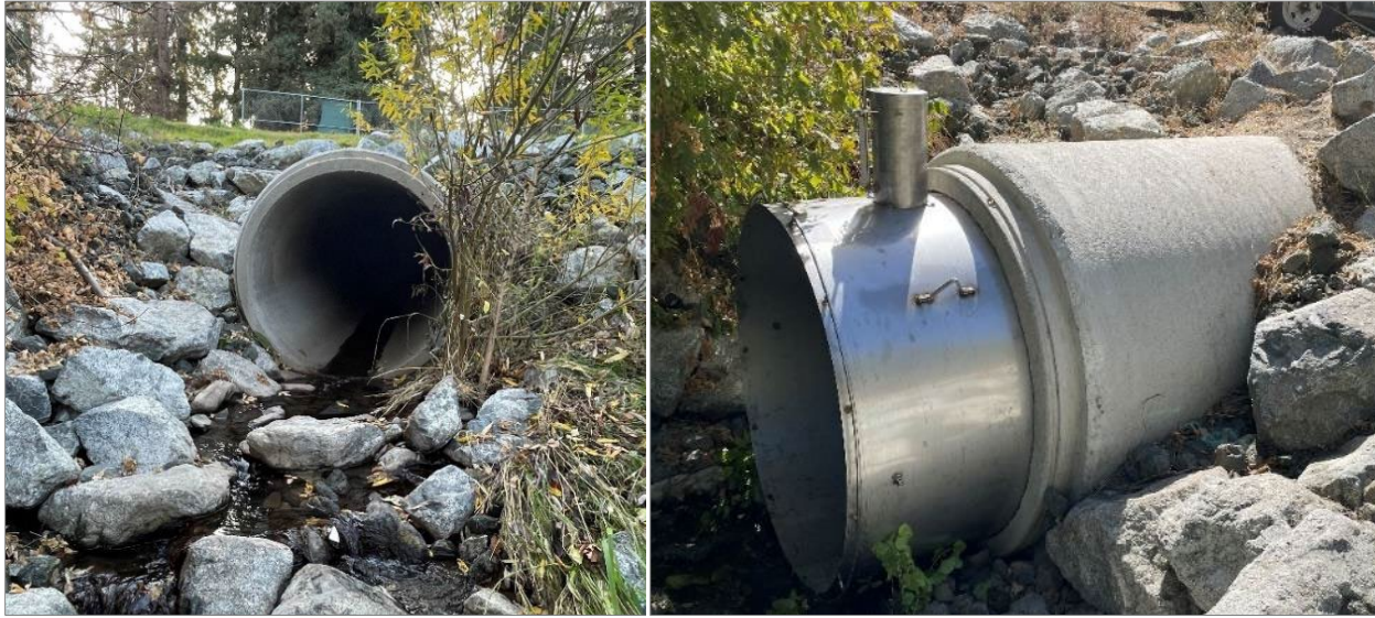
Figure SC-4. Outfall above Coyote Creek, City of San Jose
