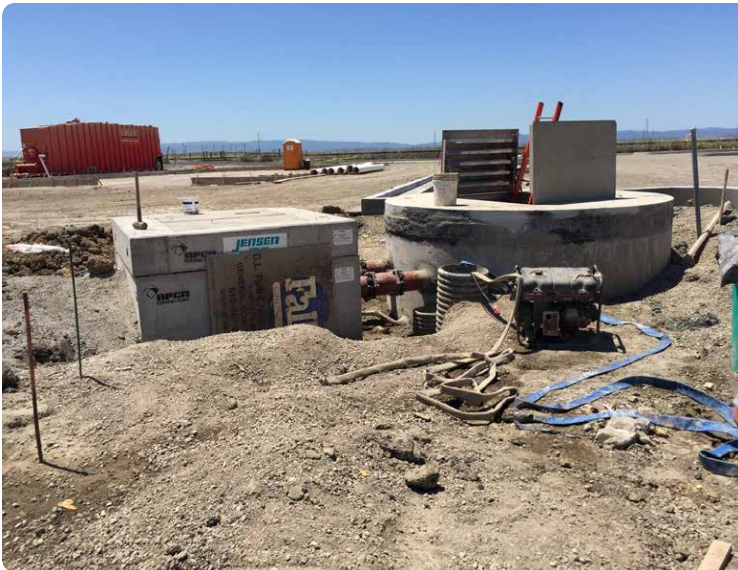
San Lorenzo Park Storm Drainage Pump Station
