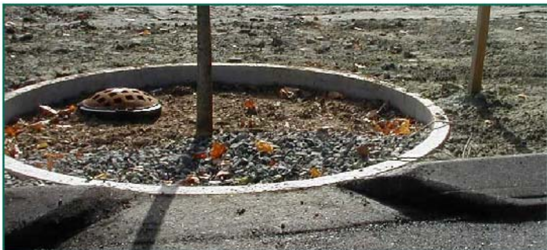
Figure 6-15: Tree Filter with Overflow Bypass. Source: University of New Hampshire Environmental Research Group, 2006
