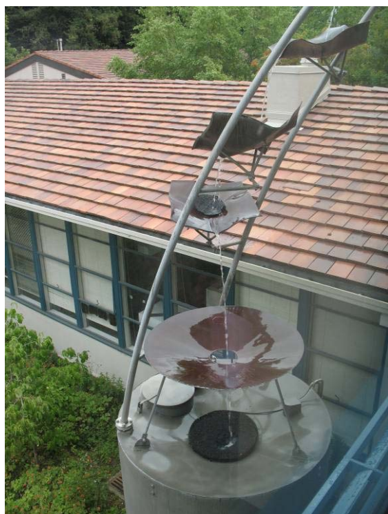
Figure 6-21: Rainwater is collected and used for flushing toilets at Mills College, Oakland.
