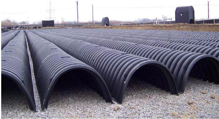
Figure 6-20: Photo of subsurface retention/infiltration system installation under a parking lot. Source: CONTECH Engineered Solutions.
