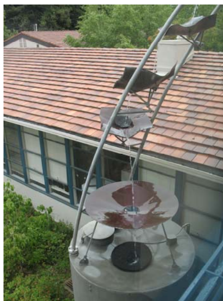
Figure 4-8: Rainwater is collected and used for flushing toilets at Mills College, Oakland.
