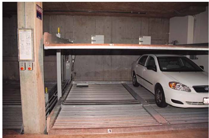
Figure 4-7: Parking Lifts in Parking Garage, Berkeley
