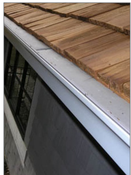
This gutter is covered by a fine mesh gutter guard to keep debris out.
