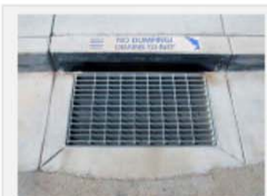
Only rain down the storm drain.
