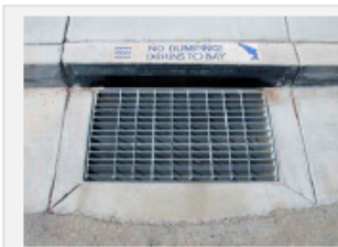
Only rain down the storm drain.
