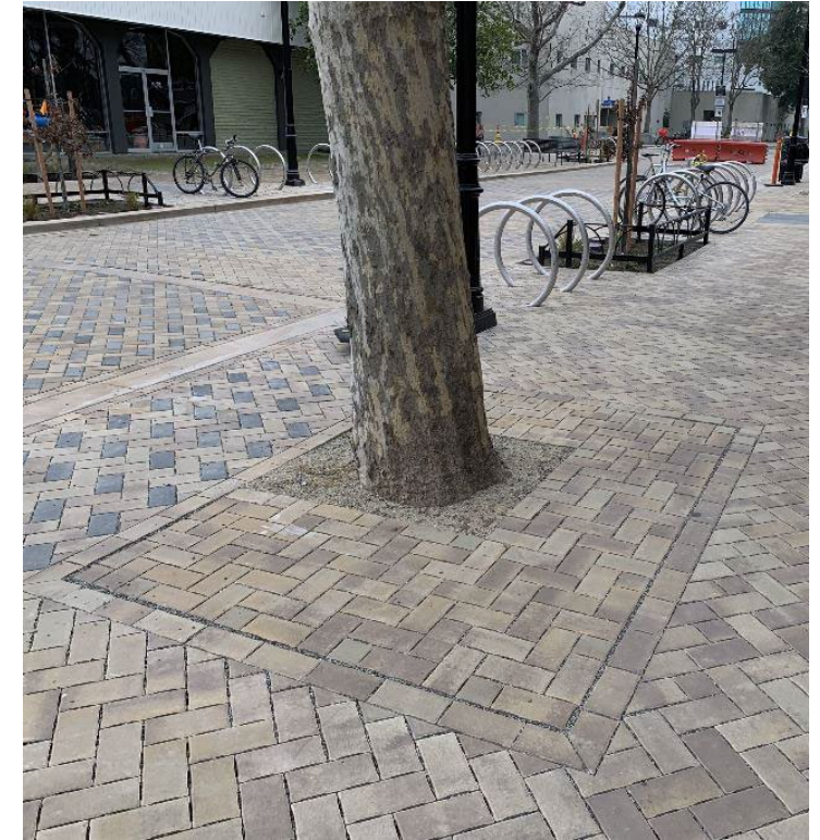
Tree Well Filter/ Pervious Pavement
