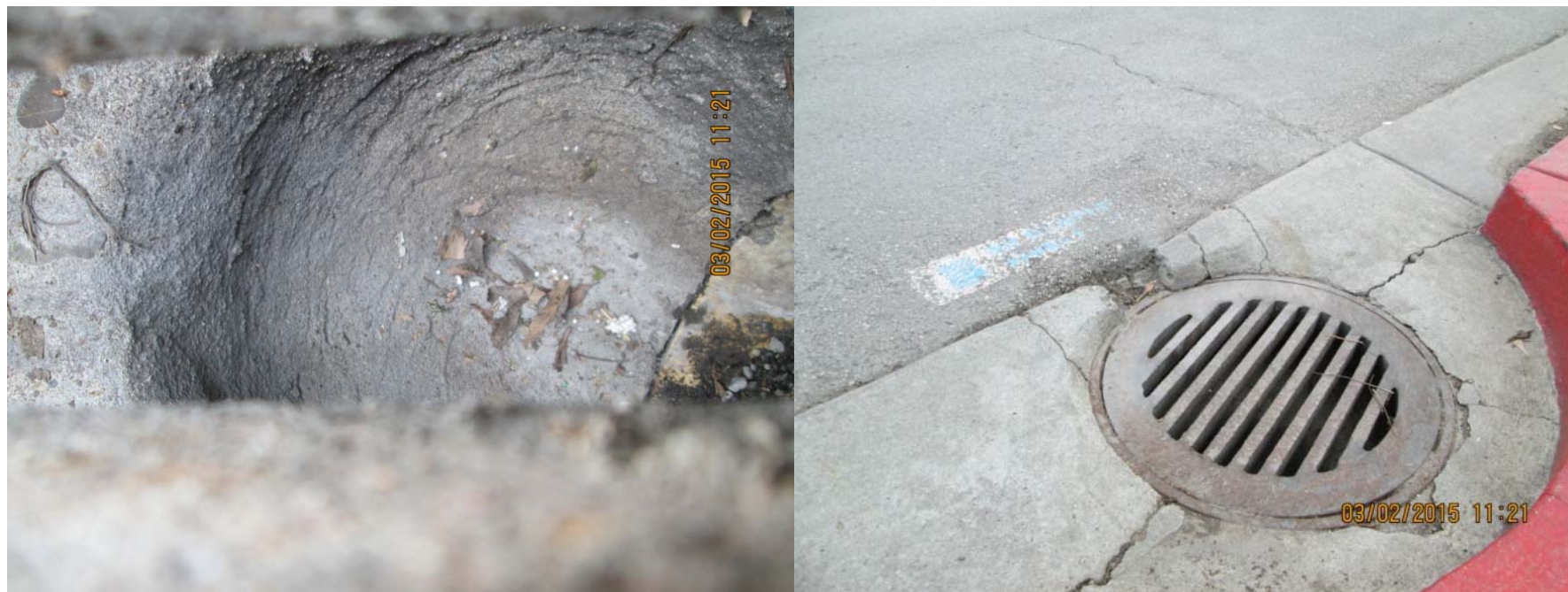
Stone cutting slurry residue removed from roadway and storm drain
