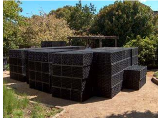
16,000 gallon, underground rainwater cistern at Rosenberg Residence, Palo Alto
