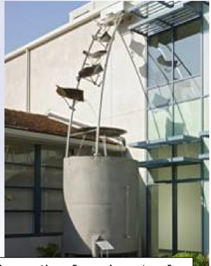
Harvesting for rainwater for indoor toilet flushing
