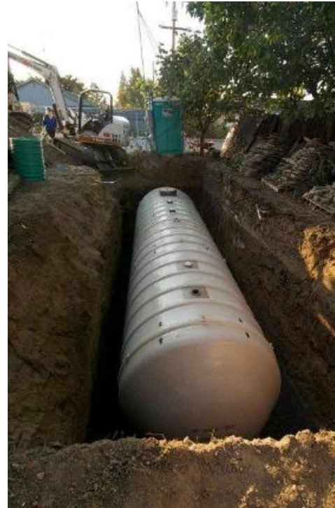
Cistern at Private Residence in Mountain View
