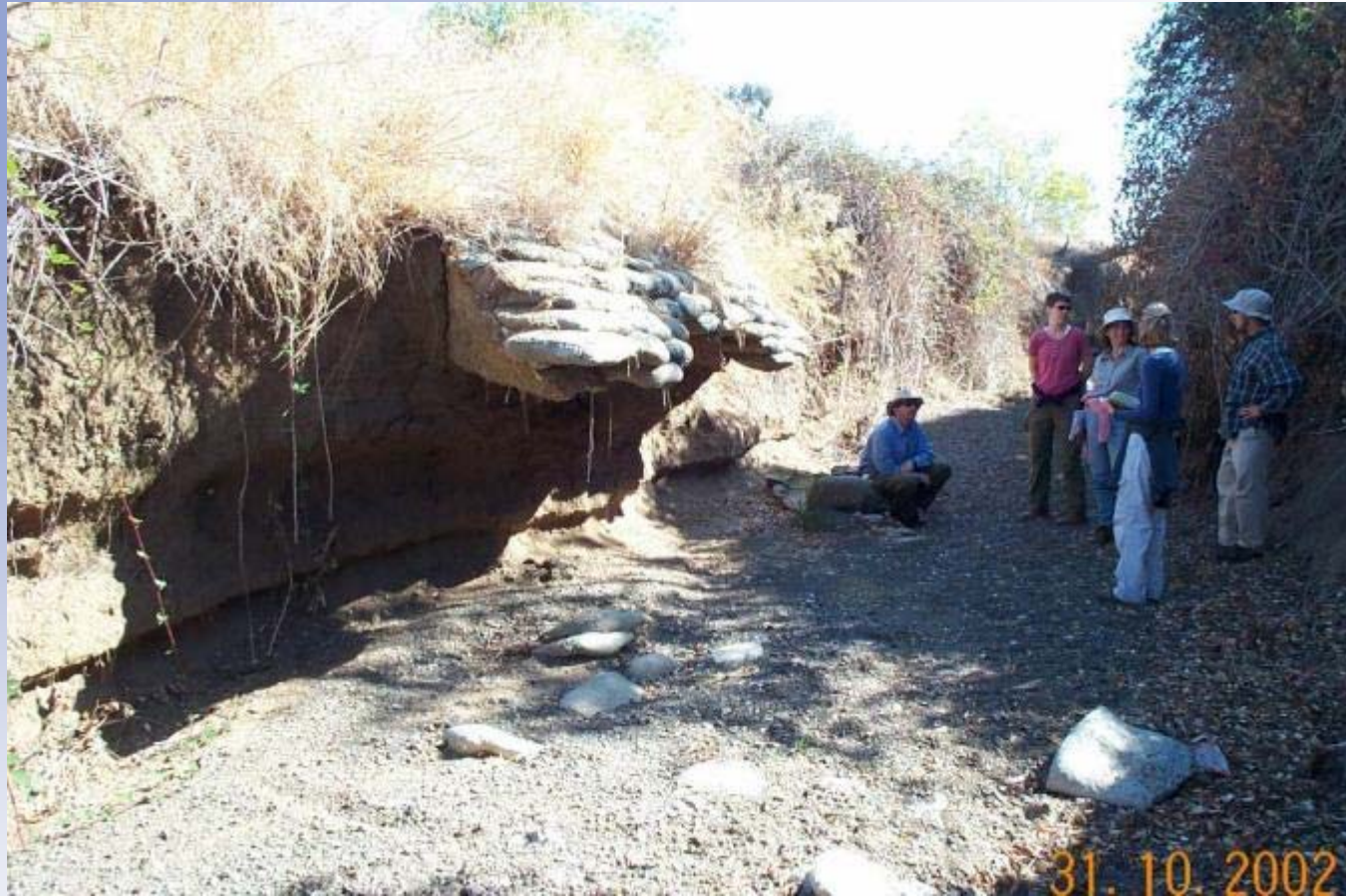
Lower Silver Creek (Erosion undermining outfall protection structure on left bank)
